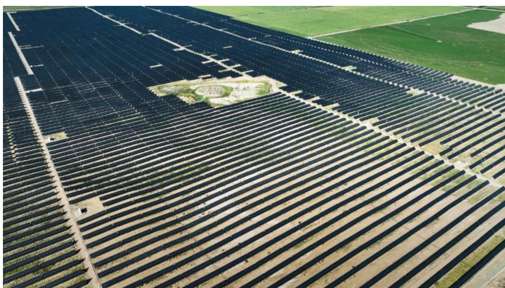
Fig.3 Solar PV Facilities
